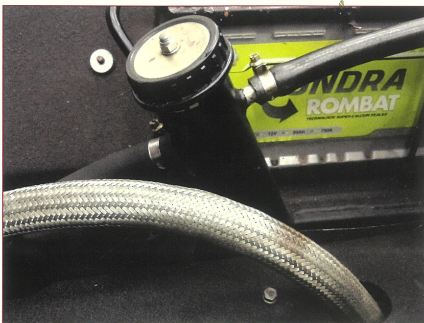
Serbatoio olio Oil tank
